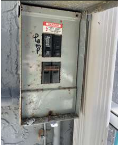
Location: POOL PUMP PANEL
