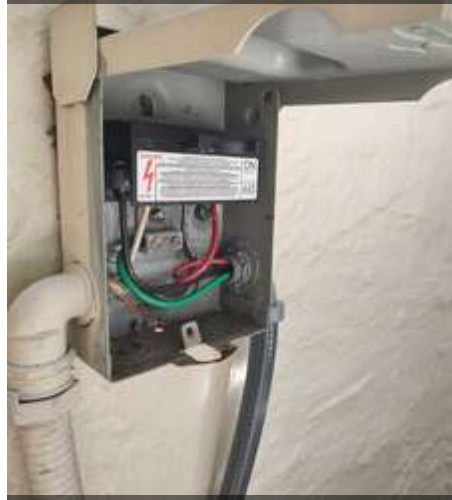
HVAC condenser unit disconnect
