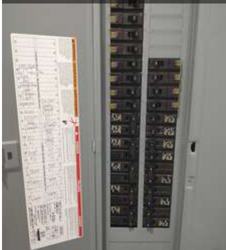
Reset for all GFCI circuits throughout the home
