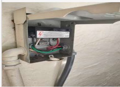
6.5.1.1 HVAC condenser unit disconnect
